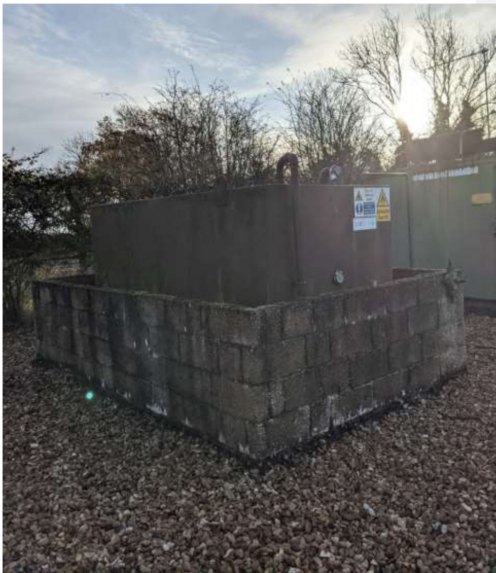
Photo 1: Waterbeach WRC fuel tank
